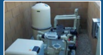
POOL & SPA EQUIPMENT REPAIR SPECIALISTS
